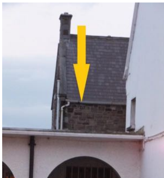
View of a section of the rear of building. Orientation is North West
