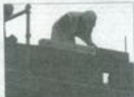
A Swift Conservation Centre worker during the construction of a new building in Mayo.
