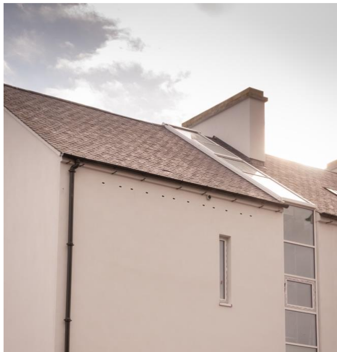
11a. NW facing rear wall of the centre with 12 built-in nest boxes
