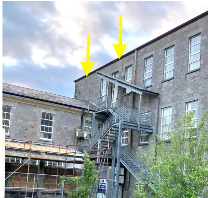
5b. SW facing – the building was reroofed and the guttering replaced in late 2023 and early 2024 but thankfully this work did not block off the entrances to the natural nest sites
